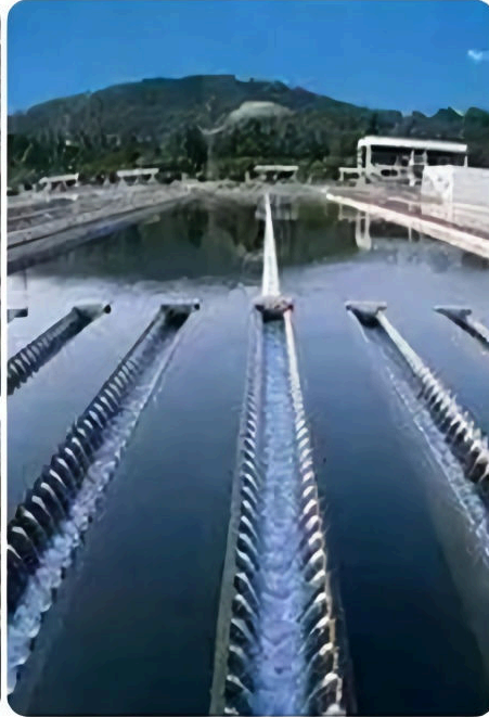
Tap water plant
